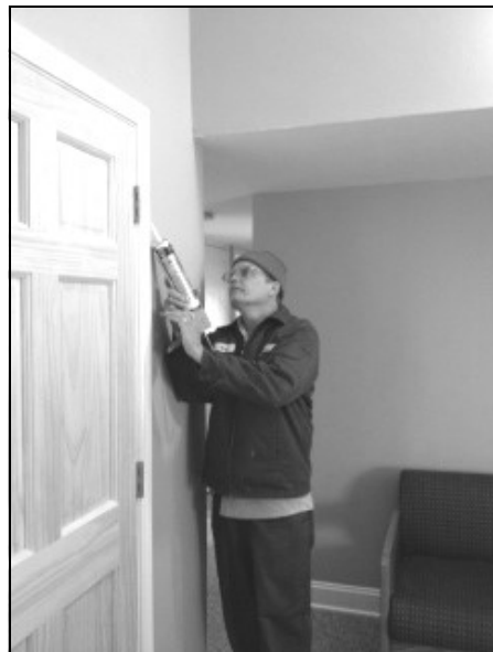
Mark Mowery performing maintenance on one of the deluxe cabins at the park
